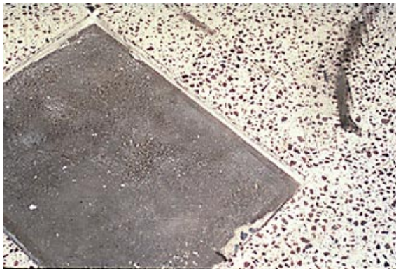
Photo 1—Epoxy Terrazzo Moisture Vapor Failure
